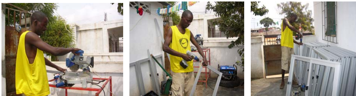
Left: Mr. A. L. is cutting a bar of aluminium. Central: He is drilling a frame of window. Right: Mr. A. L. is ensuring the screws of the windows.
